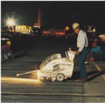
Soff-Cut International, Inc.
